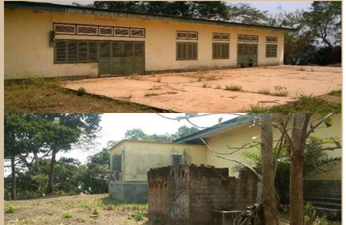
Moungoumba transit center (front and back view) before rehabilitation by AIRD CAR Program
